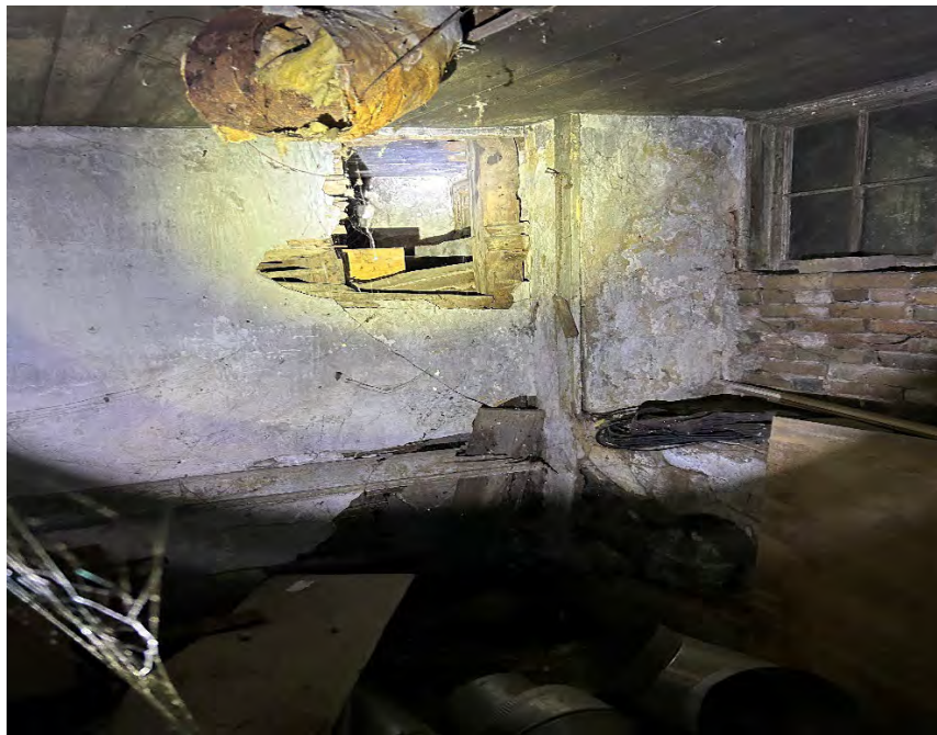
18. Damaged wall in basement of subject building.
