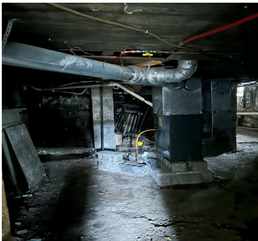
11. Basement Furnace below subject building.
