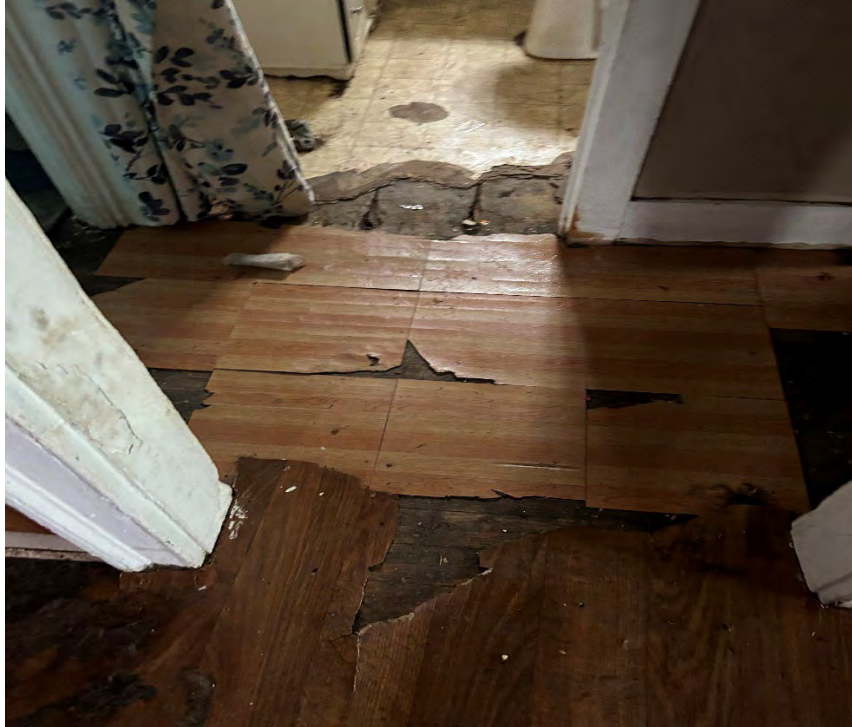
15. Damages flooring in upstairs main hallway and bathroom upstairs of subject building.
