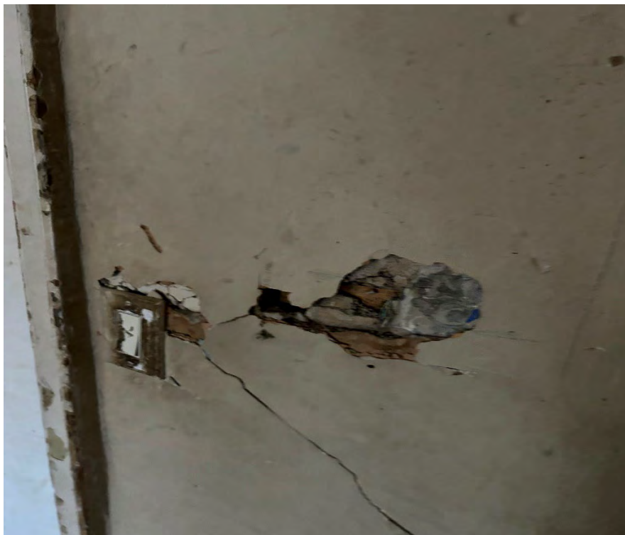
20. Damaged plaster walls in upstairs portion of subject building.
