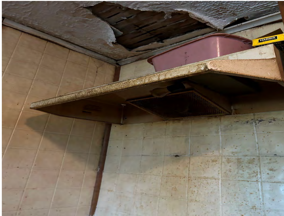
8. View of damaged kitchen ceiling.
